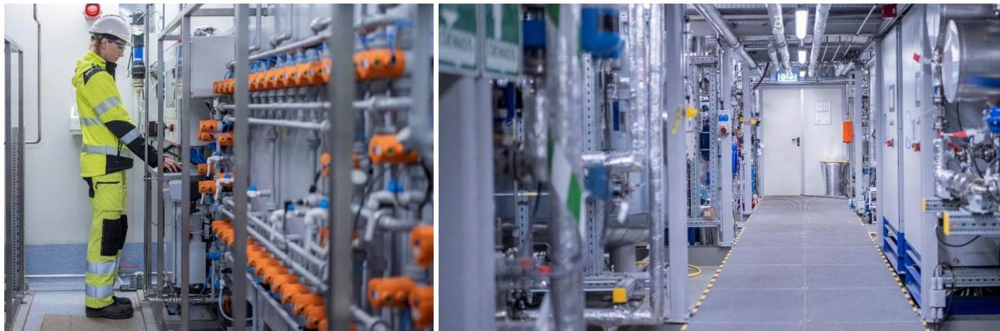
LEOP: Vulcan's operational upstream Lithium Extraction Optimisation Plant
