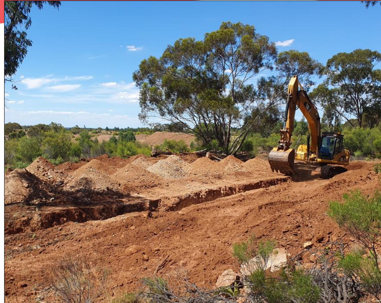
Trench T5 while being excavated – looking north towards the edge of the Southern Open Pit with the walls in background
