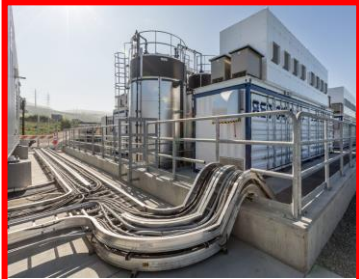
San Diego Gas & Electric (USA)
