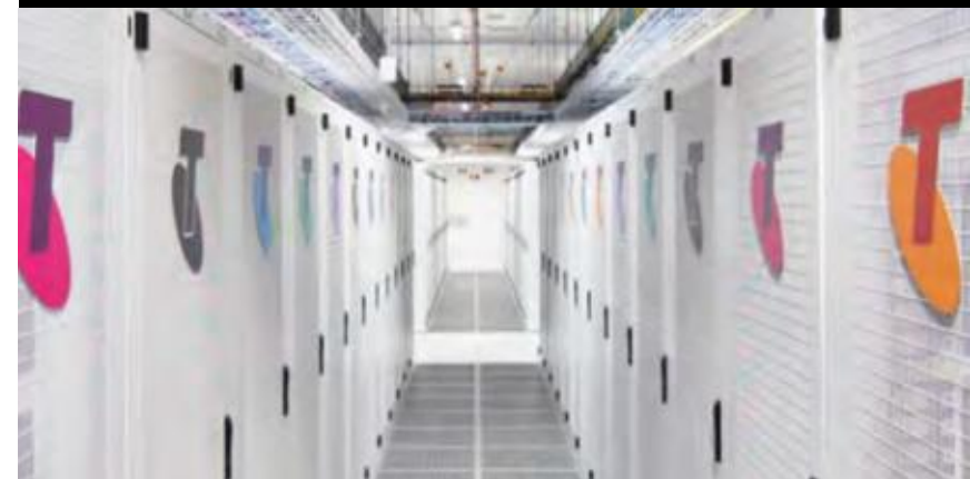
TELSTRA DATA CENTRE, CLAYTON VIC
