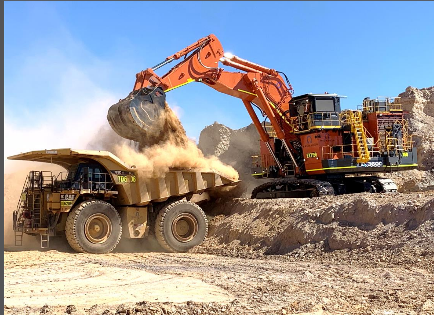
Eventual ramp up of open pit mining fleet to three excavators and sixteen trucks
