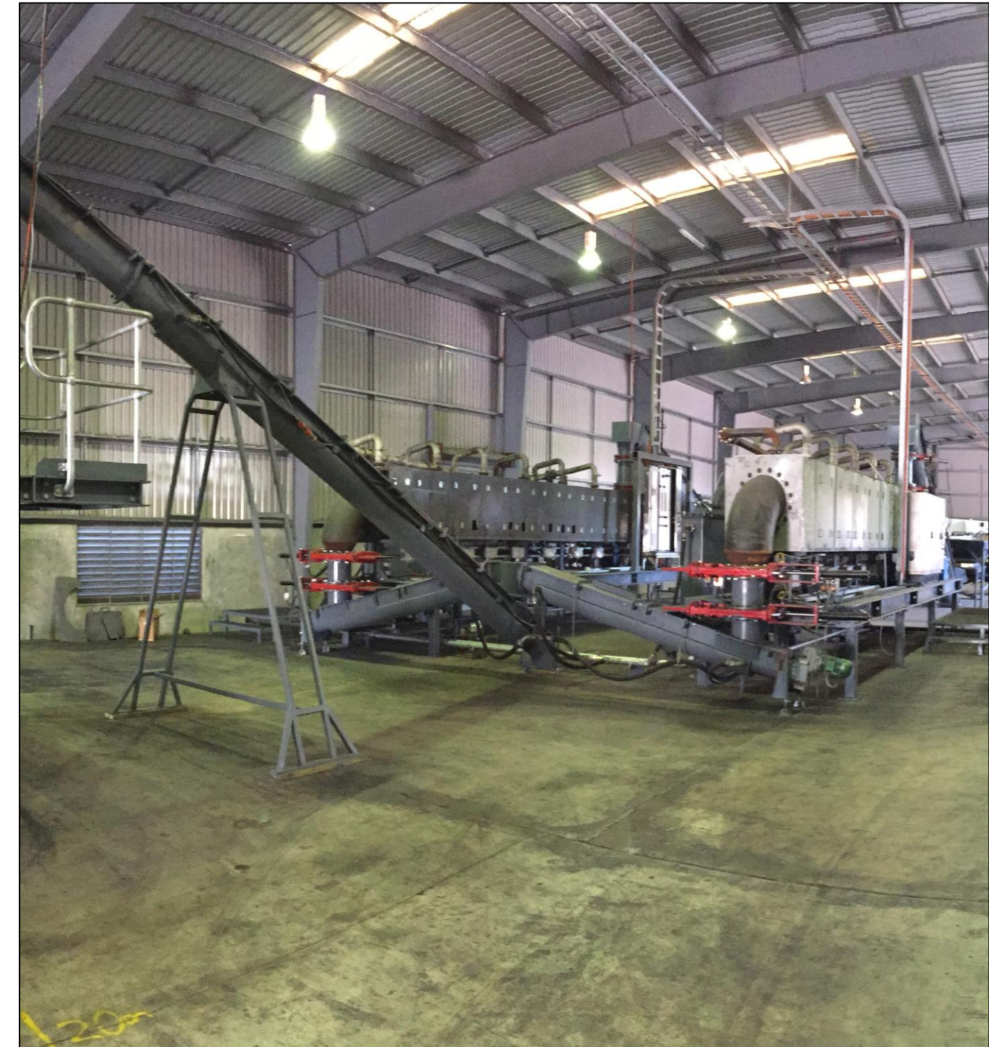
Thermal desorption units at Pearl Global's Stapylton site.
